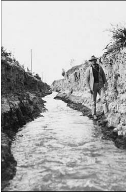
Erosion and High Velocity on the Palmetto Canal of the Imperial Canal system. Joseph Lippincott Barlow, 1864–1942, Courtesy of the Lippincott Collection, Water Resources Center Archives, University of California, Riverside.
